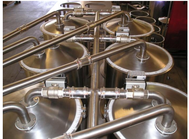
6 units group from above
