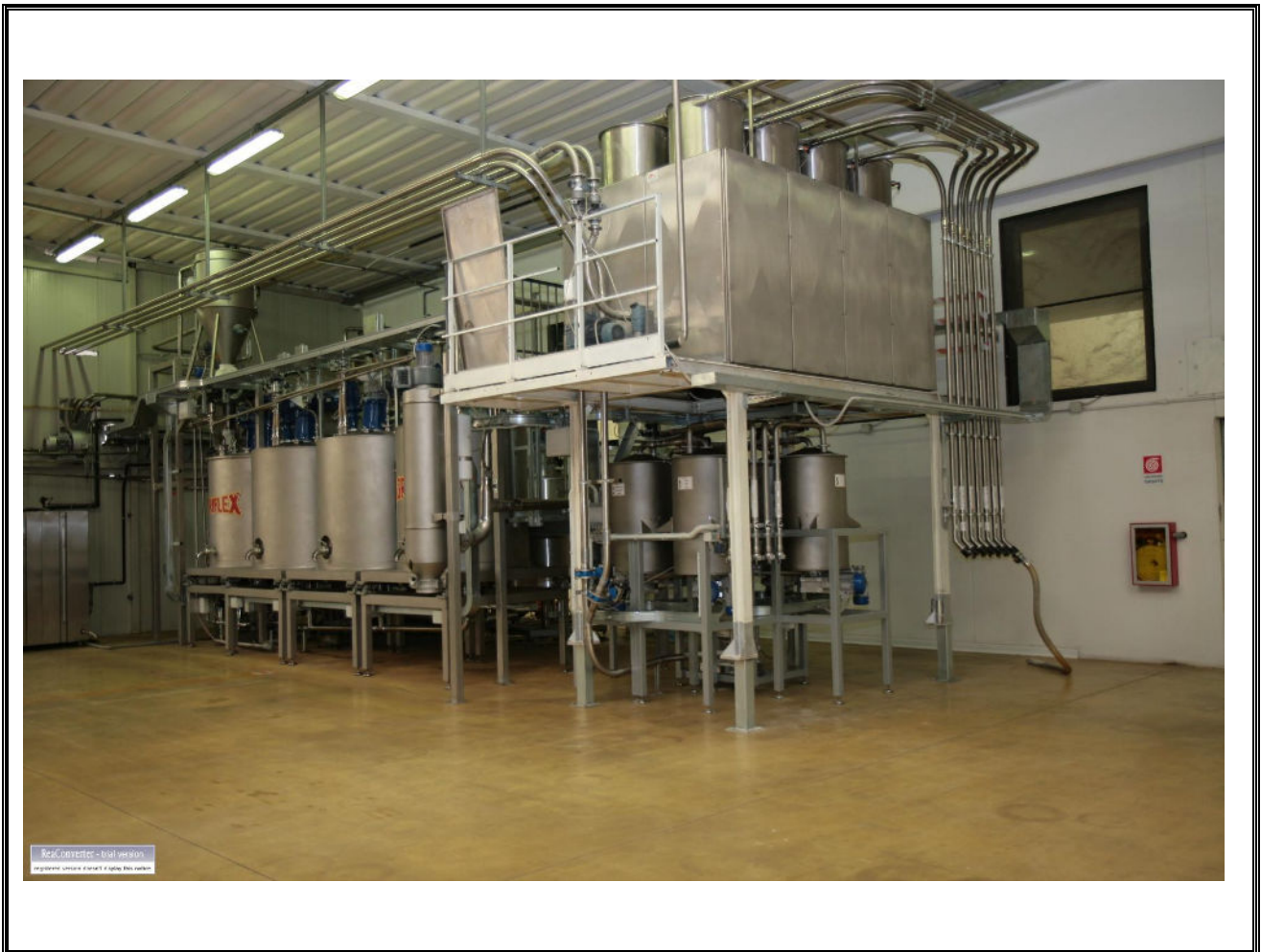
Installation with pneumatically-charged micro-ingredient station and automated system for natural yeast dosing
